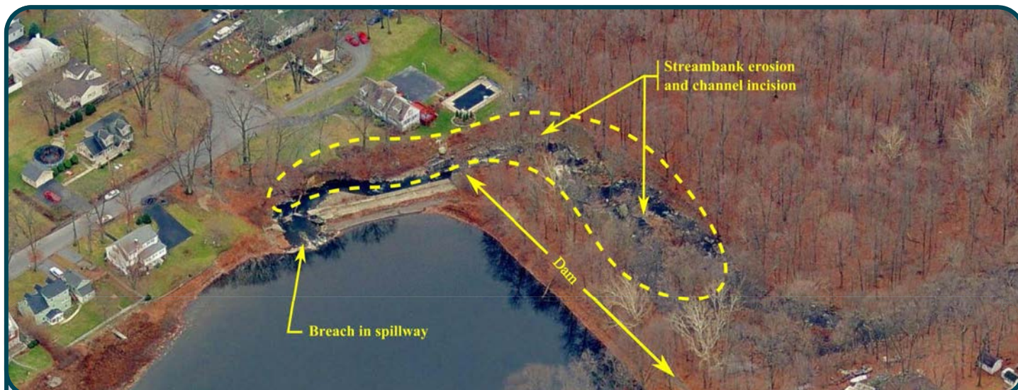
Figure 1: Aerial view of Winona Lake spillway breach and affected area. Stream flow patterns after the breach have caused undercutting of the back side of the dam, streambank erosion that is encroaching upon a neighboring residence, and incision of the stream channel.
