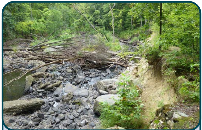
Photo 1: Streambank erosion along the down stream side of the Winona Lake dam, photo courtesy of Ted Kolhmann. Undercutting of the dam shown on the right.
